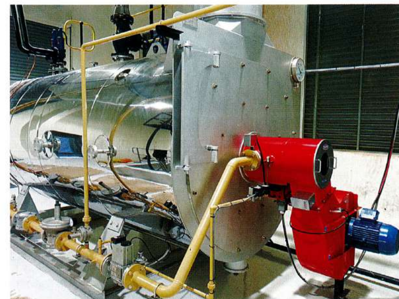
The first Cyclotherm boiler with a Limpsfield Gas fired burner and auto flame combustion control system in South Africa
