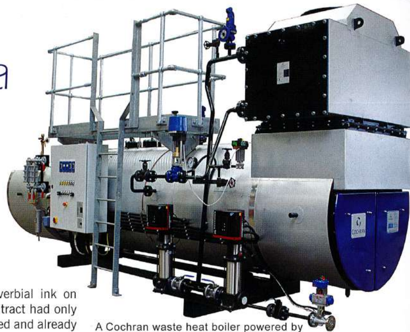
A Cochran waste heat boiler powered by exhaust of a gas-fired electric generator
