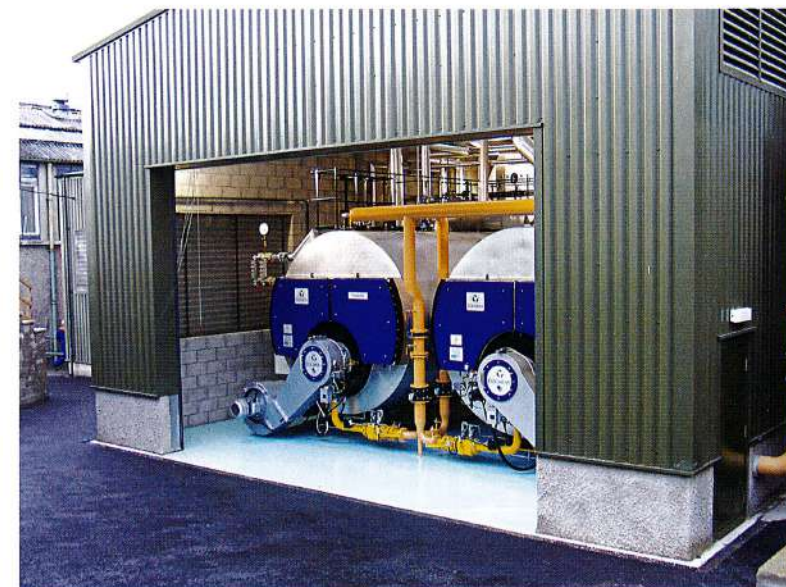
Two Cochran 10T Thermax gas fired boilers installed
