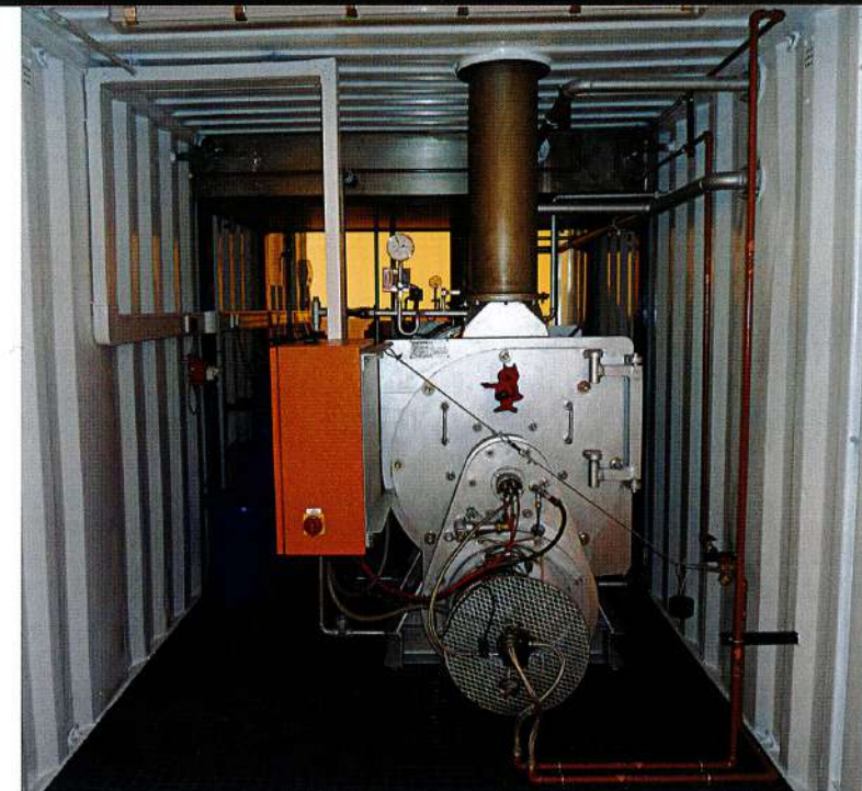
A mobile steam plant with containerised boilers
